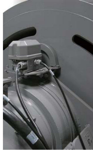
Upper and lower hoist limit switch
